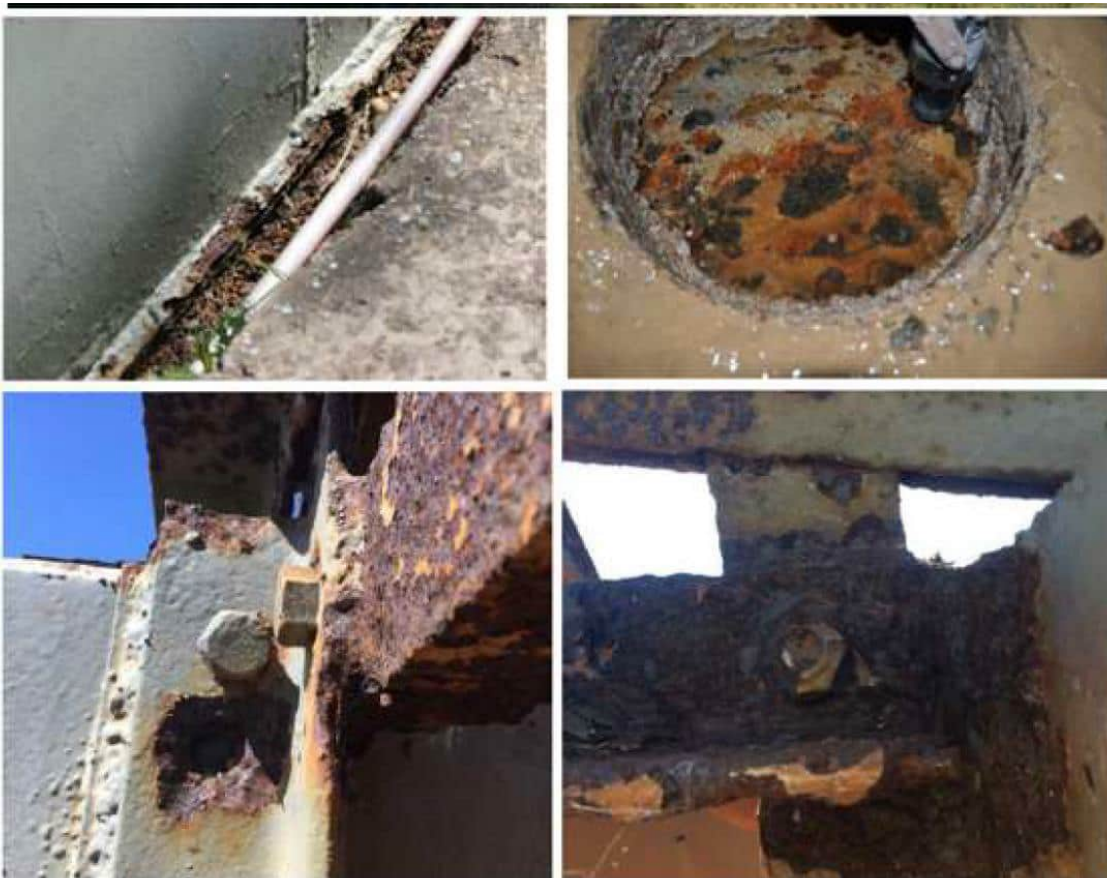
Photo 2-1 Harpers Hill Reservoir defects. Source (Hunter Water, 2021a)
