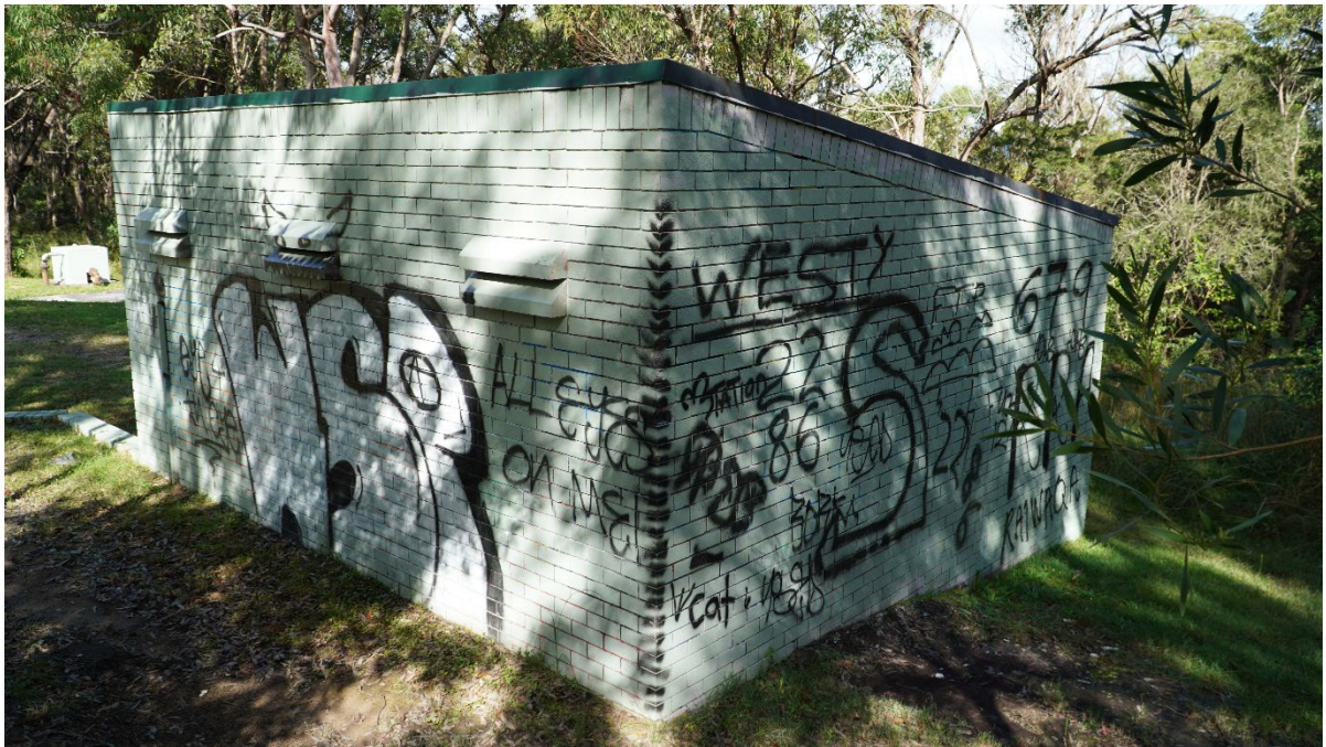
Plate 9. View south-west at the southern and western side of the pumping station building.
