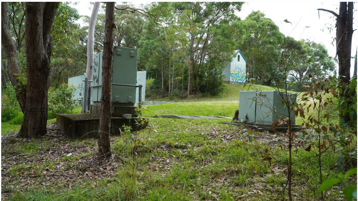
Plate 12. View north-east towards a pumping set, 15m south of the 1980s Pumping Station Building, and 30m south-west of the valve house.
