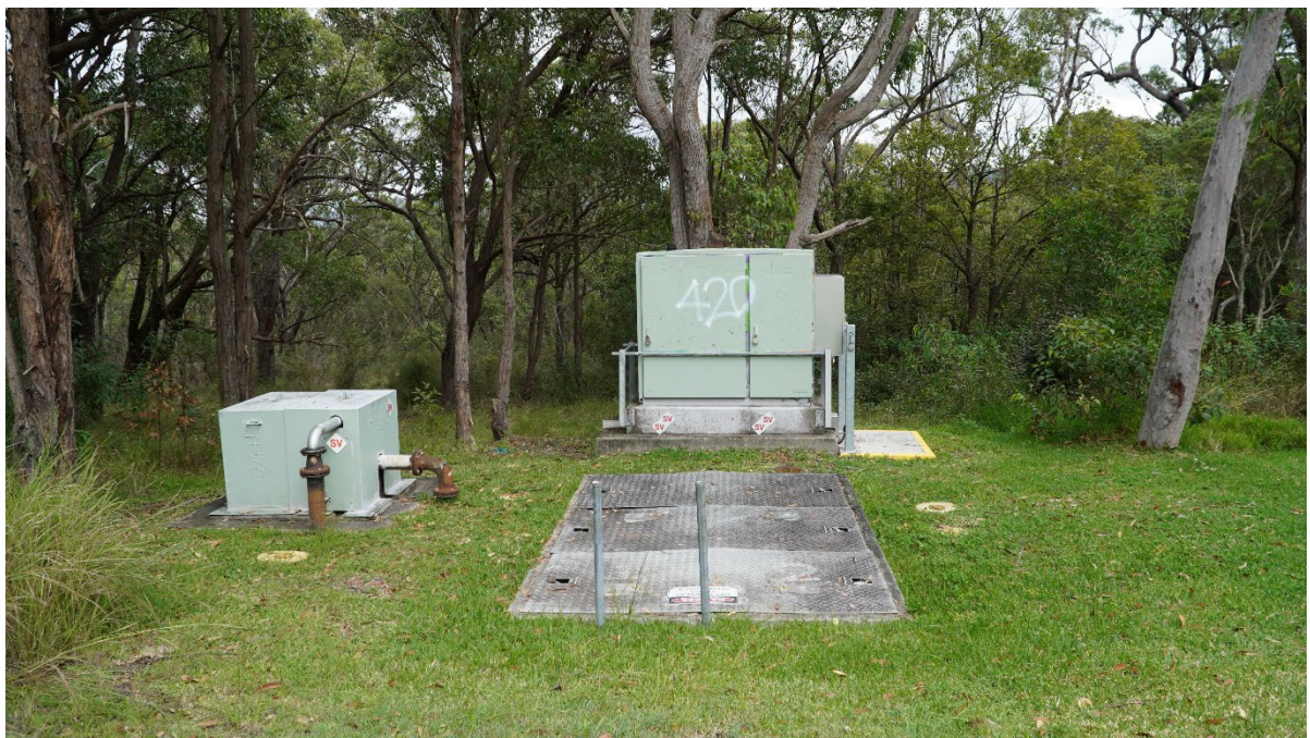
Plate 13. View south at pumping set infrastructure, including a pit covered with a metal grate.
