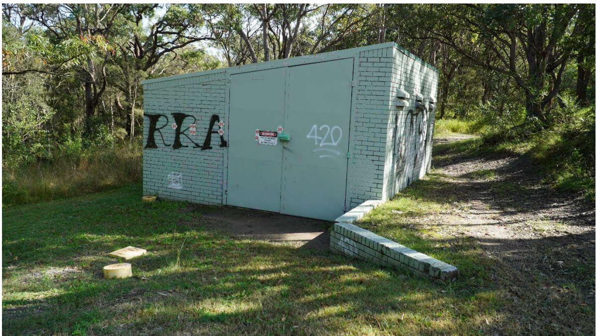
Plate 10. View of the southern side of the building, showing the concrete landing, metal entrance doors and a small retaining wall
