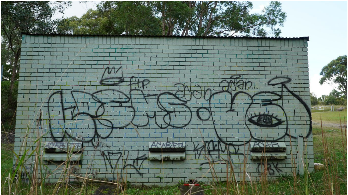
Plate 11. View of the western side of the building, showing two concrete open drains and three vents, with a 30cm scale.
